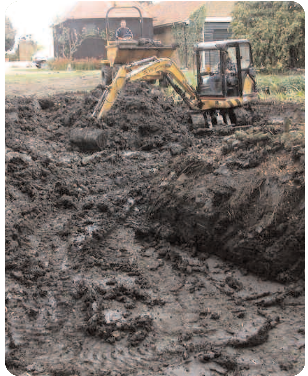
Digging pond by machine. Depending on the size of your pond, you can dig it by hand or machine.
